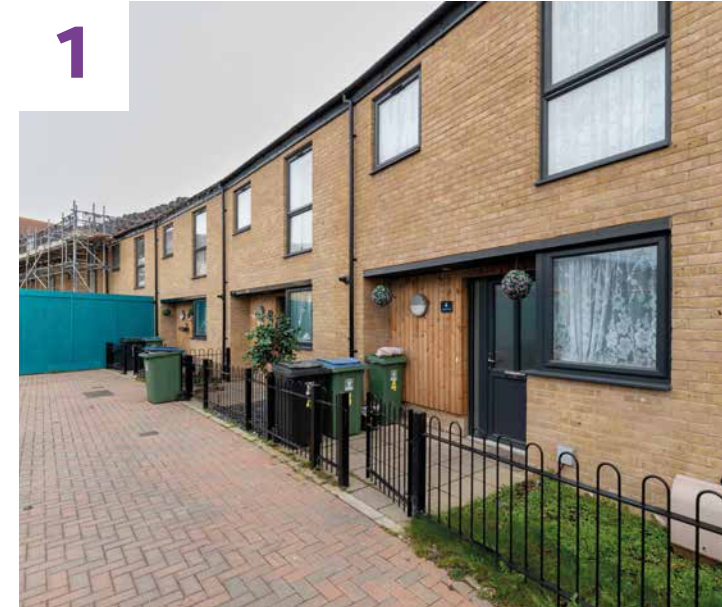
Work is progressing well on the homes at Kingfisher Way and The Turnstones, with the scaffolding completely removed now, the roofs in place, and landscaping well underway.
